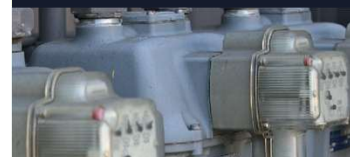
Water Metering and Utilities
