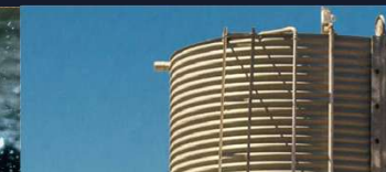
Tank Level and Quality
